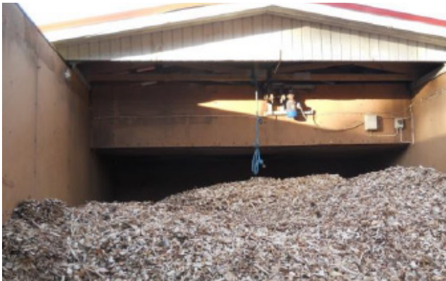
300kW heating plant
