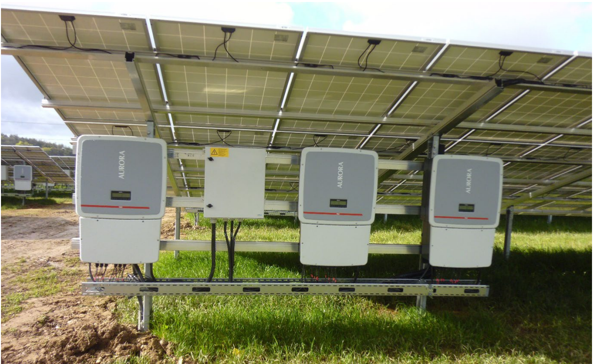
Example of solar farm string inverters. Image provided by Local Power Ltd
