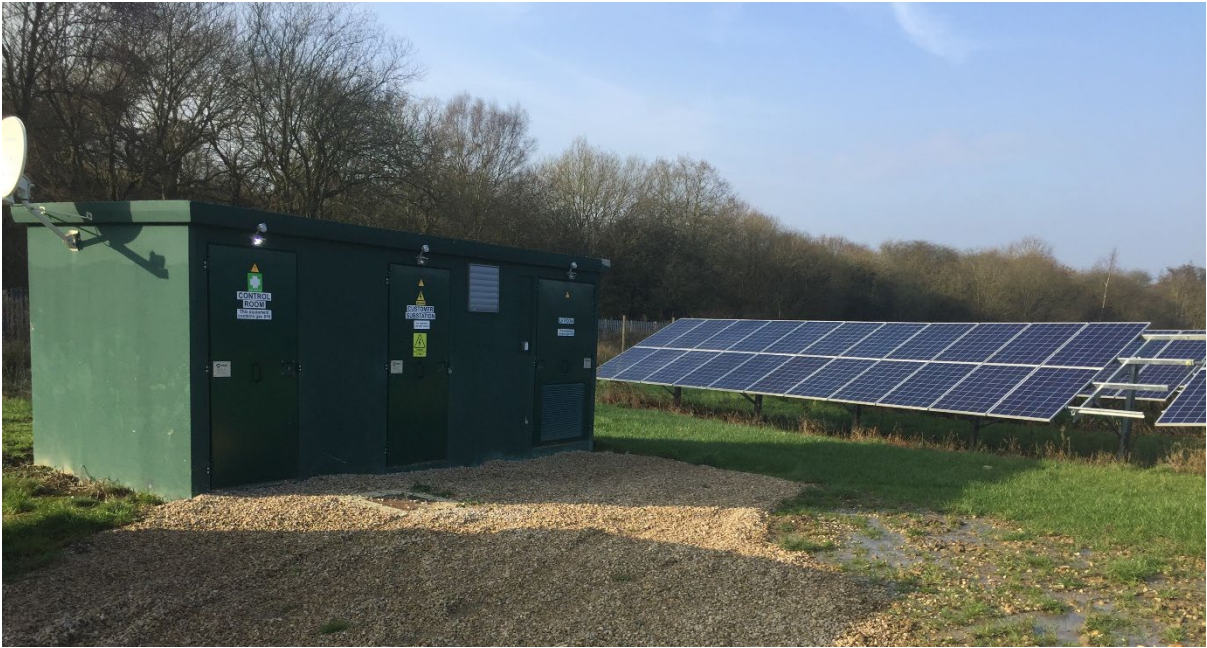
Solar Farm customer and network operator substation – existing tree/hedgerow boundary and stock proof perimeter fence visible in background. Image provided by Local Power Ltd.
