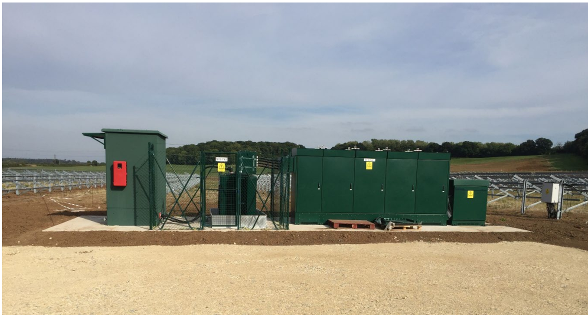
Solar Farm Inverter and Transformer Station, panel mounting System in the background – image provide by Local Power Ltd.
